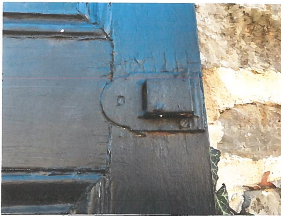
Figure 4. Example of shutter wood cracking and buckling. Buckling results when increased moisture conditions cause the wood to expand.
