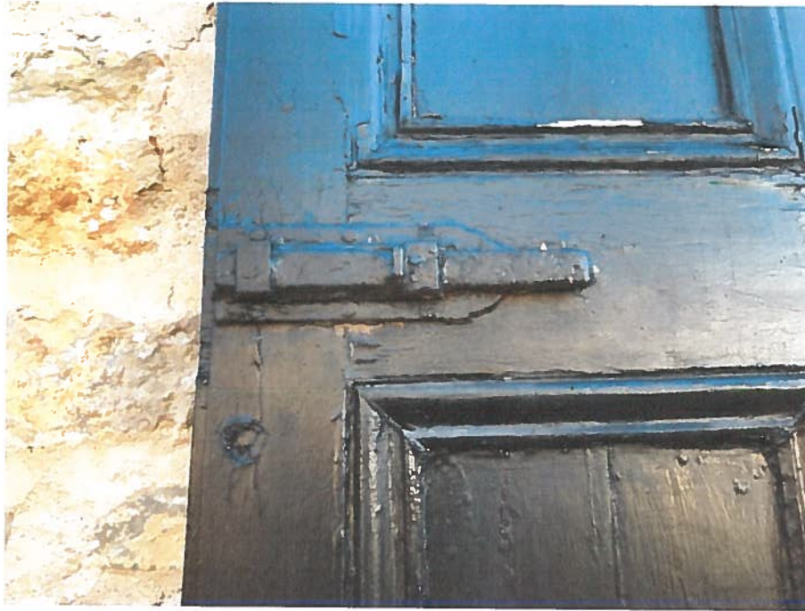
Figure 5. Examples of wood cracking, chipping and buckling due to prolonged exposure to the elements. Shutters were likely painted in slap-dash manner, i.e. overtop of aged wood and paint surfaces, rather than sanding to a relatively fresh, clean surface.
