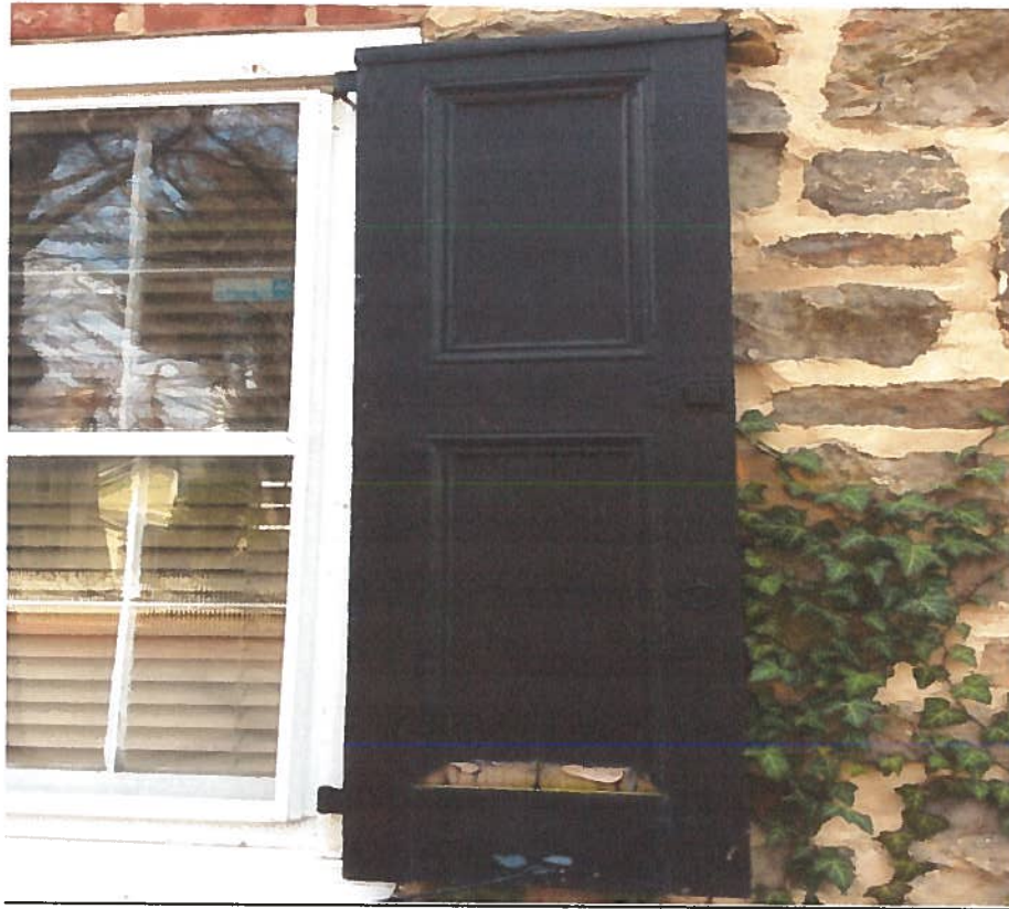
Figure 3. Missing wood piece from 54 E Wall St shutters
